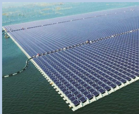
Fig. 1: Floating Solar Panel
